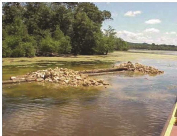
Figure 5.9. Rock-log breakwater at Peterson Lake, Pool 4, Upper Mississippi River. Photo credit: USACE, Rock Island District.
