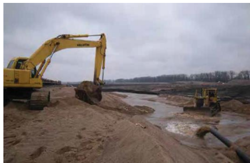
Figure 9.3. Dredging may be necessary to maintain or create connections between the reservoir and water bodies in the floodplain. Photo credit: U.S. Army Corps of Engineers (USACE), Rock Island District.
