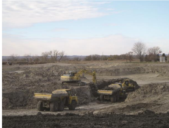
Figure 3.10. Excavation of accumulated sediment at a Nebraska reservoir. Photo credit: M. Porath, Nebraska Game and Parks Commission, Lincoln.
