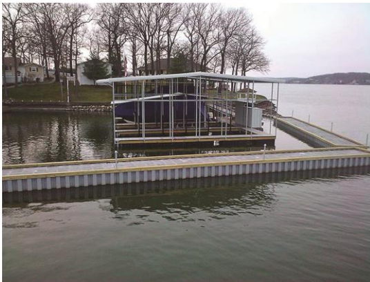
Figure 5.12. Pontoon-type breakwater. Photo credit: Horseshoe Bend Docks and Rip Rap, Lake Ozark, Missouri.
