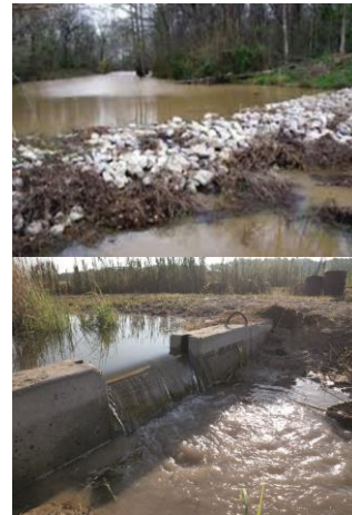
Figure 9.6. Weirs installed to retain water and prevent premature dewatering of backwater areas. Photo credit: USACE, Rock Island District (upper), and R. Kröger, Mississippi State University (lower).
