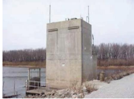
Figure 9.7. Permanent pumping station at the Andalusia Refuge, Pool 16, Upper Mississippi River. Photo credit: USACE, Rock Island District.
