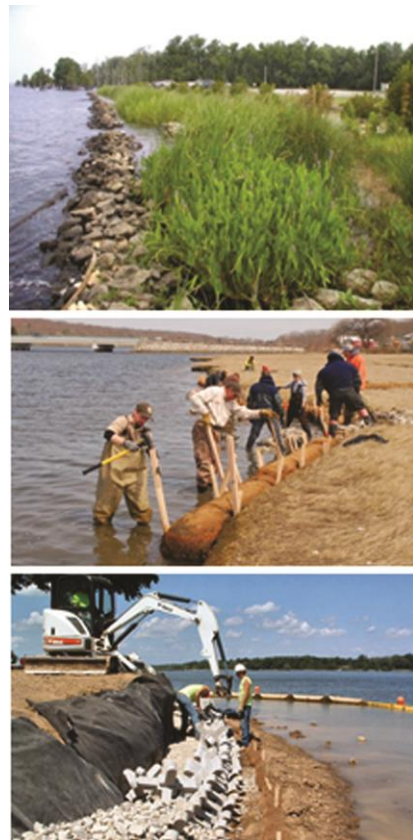
Figure 8.5. General approaches to bank stabilization include live planting, bioengineering, and hard armoring. Photo credits: U.S. Army Corps of Engineers, Savannah District (upper and lower photos), and The Nature Conservancy, Rhode Island (middle).
