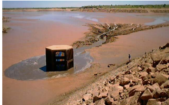
f. Reservoir sedimentation has buried the outlet at Sumner Dam near Fort Sumner, NM.
