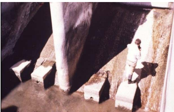
n. Sand has abraded the spillway at the Milburn Diversion Dam near Sargent, NE.
